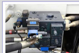
Oil Preheating System
